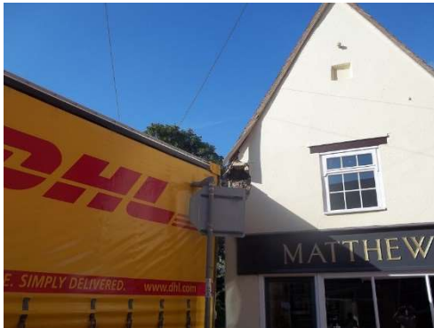
This lorry struck and damaged the building. The 6'6" restriction was ignored.
